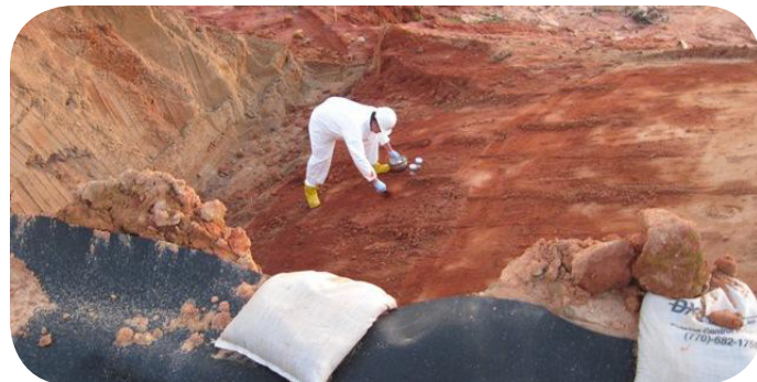
Worker collects soil samples to confirm that soil left onsite is clean.
